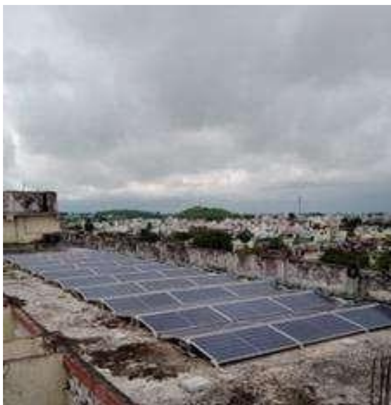
Roof top solar panel system
